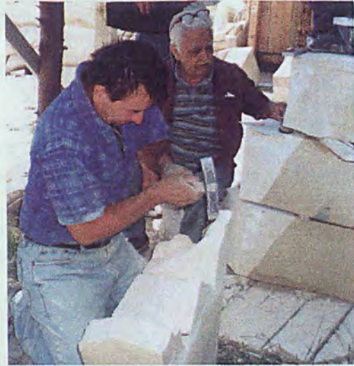
Chief craftsmen Omer Karaahmet and architect Fatin Uluengin are working on decorative elements of the minaret
